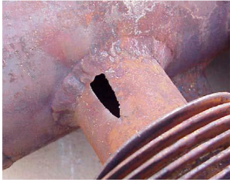
Fig. 1 – Damaged evaporator pipe
