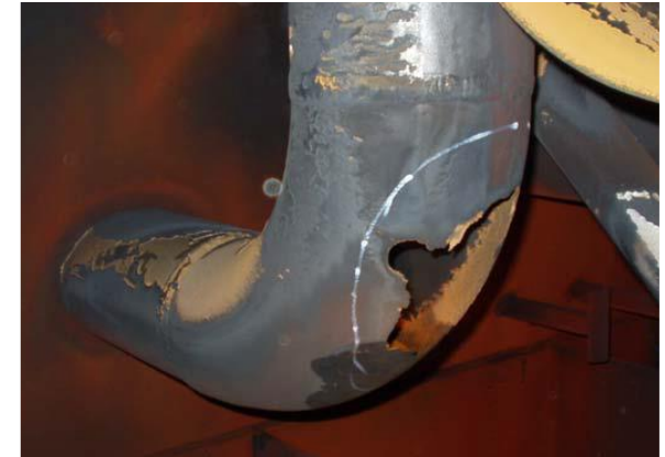
Fig. 3 – Damaged downcomer of low-pressure circuit
