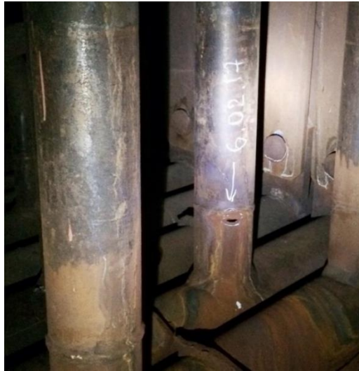
Fig. 2 – Damaged low-pressure evaporator riser on welded seam of Kirishi state district power station
